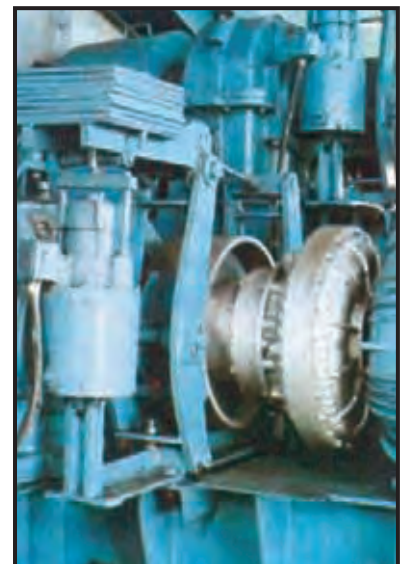
ELECON Fluid Coupling installed with Crusher drive at Gandhinagar T.P.S.
